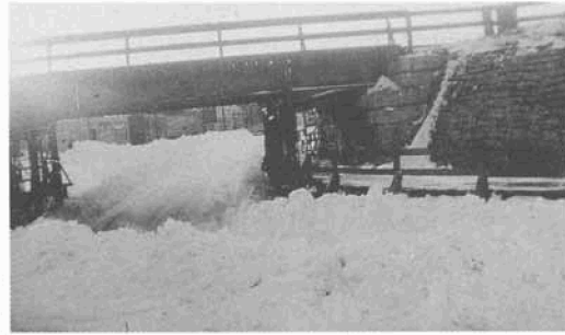
The Elma viaduct filled with snow.
