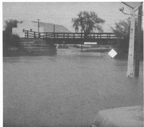
Later years, the viaduct flooded.
